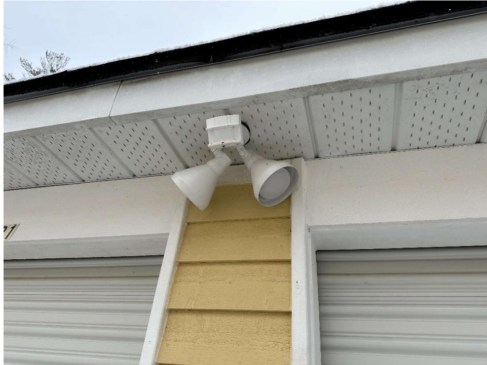
Photo 27 Soffit-Mounted Light Fixture with Motion Sensor at Storage Building
