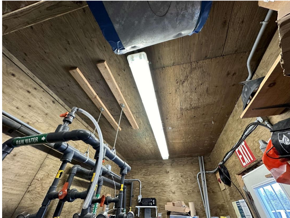
Photo 26 Ceiling-Mounted Light Fixture at Pump House
