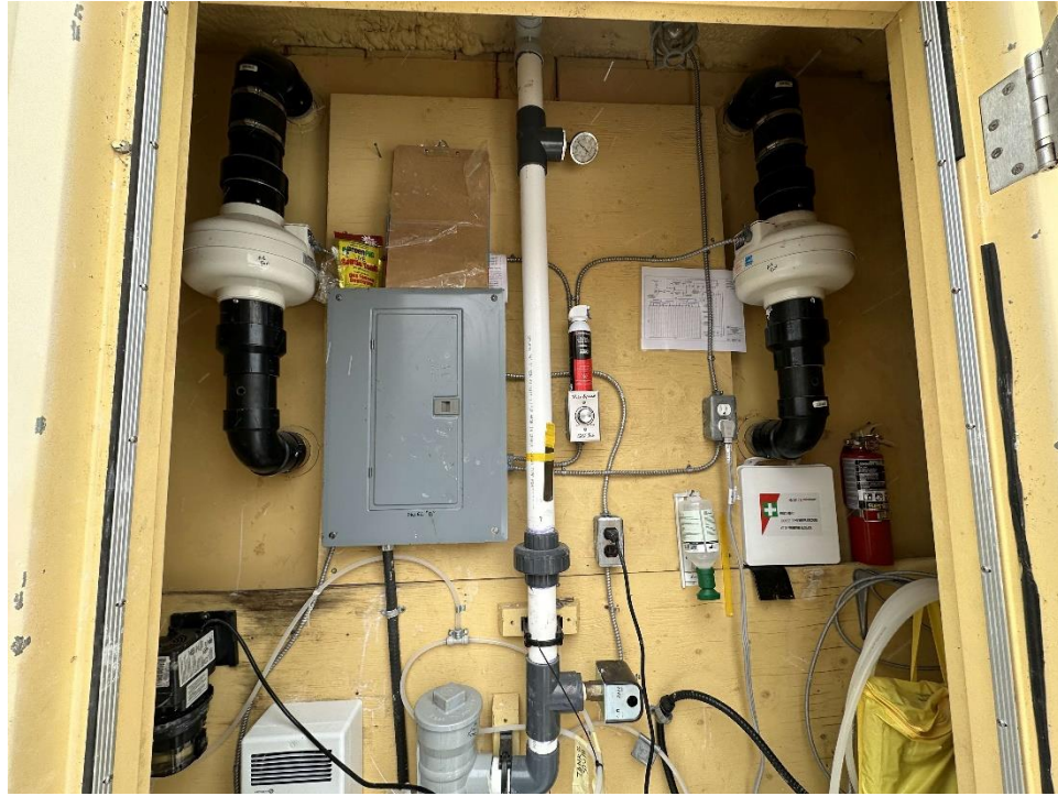
Photo 25 Distribution Panel at Waterloo Biofilter
