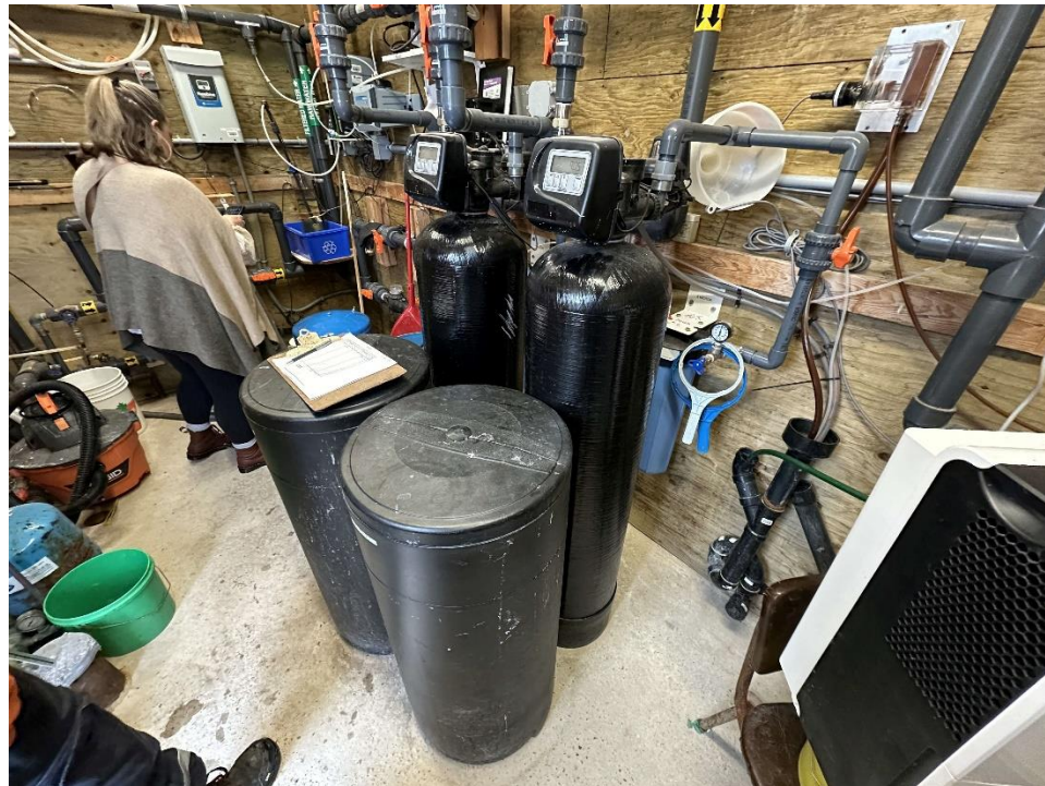
Photo 20 Water Treatment System Overview
