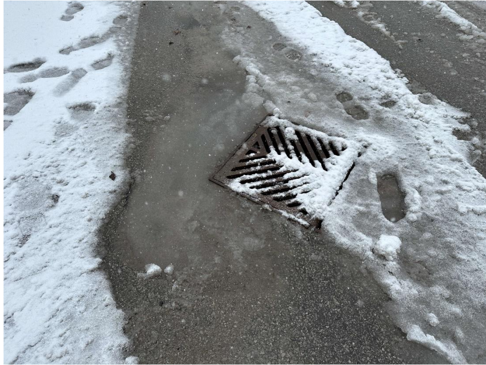
Photo 3 Localized Asphalt Settlement at Catch Basin
