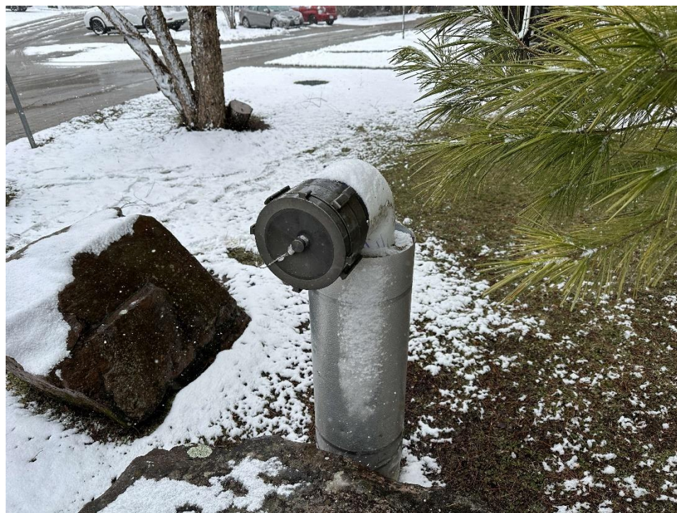
Photo 30 Dry Fire Hydrant for Fire Department
