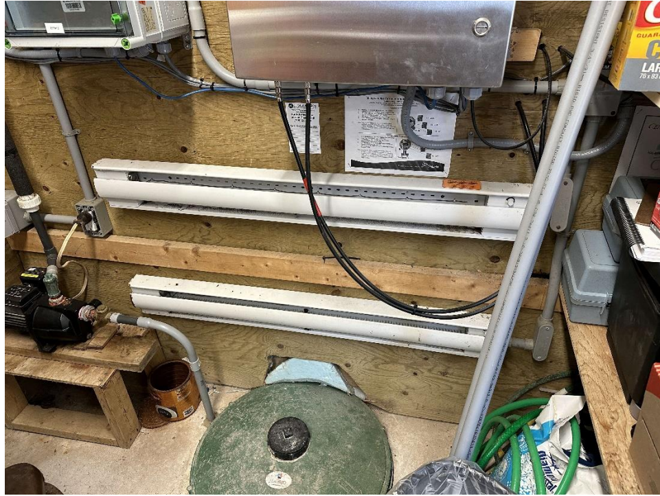
Photo 23 Electric Baseboard Heaters at Pump House
