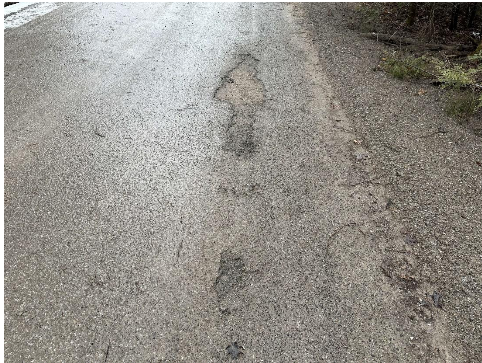
Photo 2 Localized Potholes on Main Roadway
